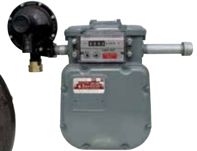
Attached to Vapor Meter
